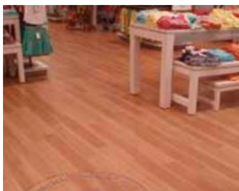
Solid Timber Flooring installed over Ultraplan Eco in a Pumpkin Patch store in Sydney, Australia
