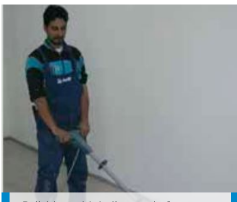
Polishing with helicopter before applying Ultraplan Eco - Mirabello kindergarten - Cantù (Como) - Italy
