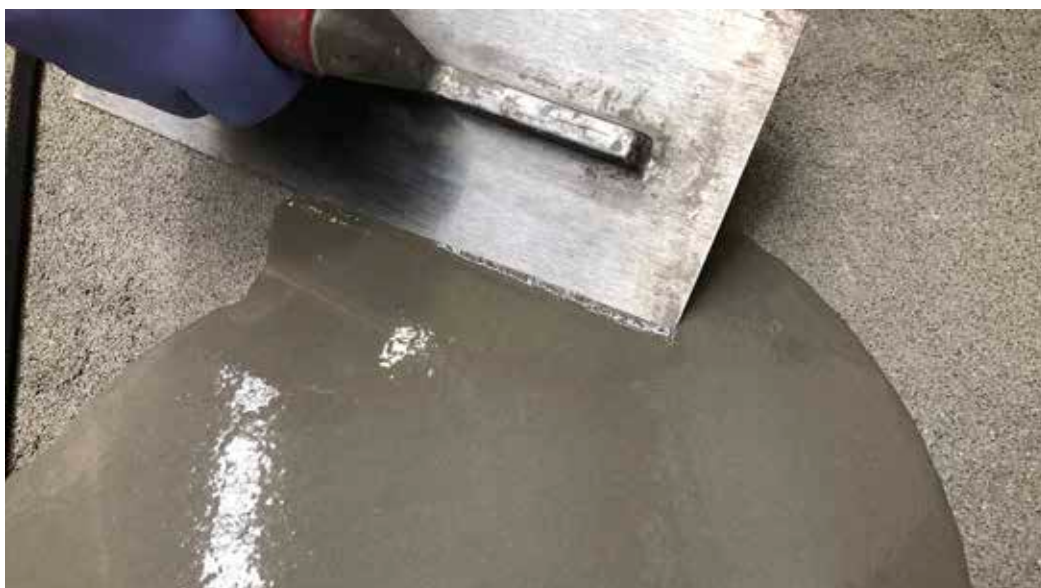
Installation of Ultraplan Trade after first priming the porous concrete substrate using Eco Prim T Plus diluted 1:2 with water
